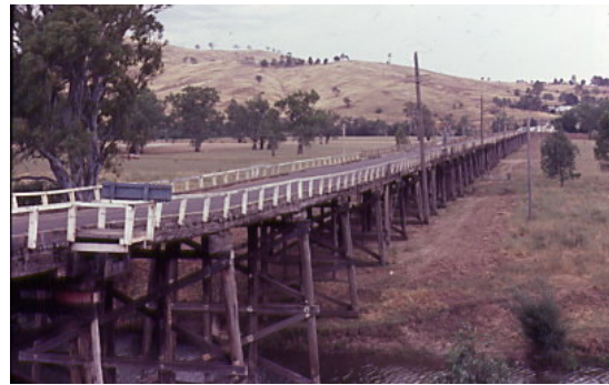
Gundagai's famous Prince Alfred timber road and rail bridge Photo by Heritage Branch
