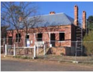
Teacher's House before and during restoration works. Images Sinclair Croft, Bathurst City Council.
